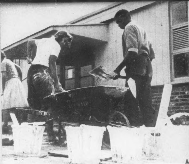
WORK CAMPS sponsored by Quakers are designed to give young people a taste of how less fortunate live. At Fanner House in Indianapolis, campers paid $35 a month for privilege of cleaning some 200,000 bricks and constructing new buildings. Here are two work campers mixing mortar for a new health center. A housing project for 400 families is now being planned.
